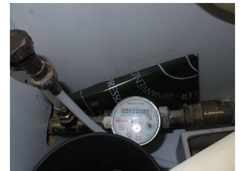
Messingfitting i rustfri installation
