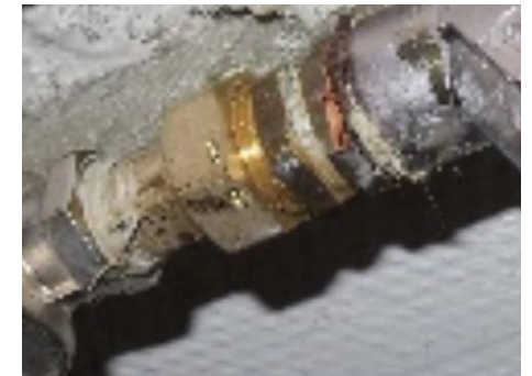
Messingfitting i rustfri installation
